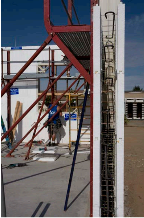
End view of a PolySteel wall waiting to be filled with concrete August 08
